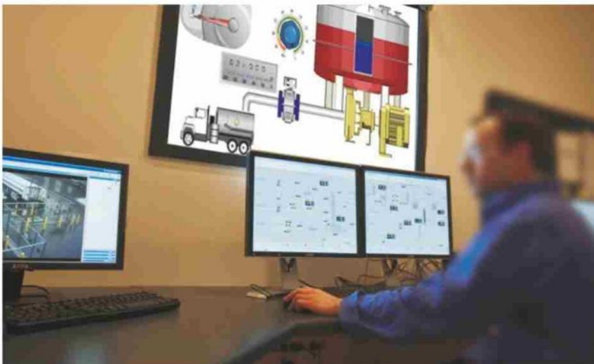
Wall mounted 19" and above, HMI
